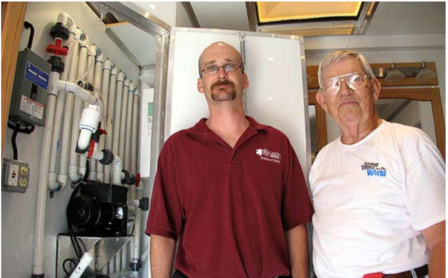
Mike Moore (center), Carolinas MED1 maintenance specialist, and LWW's Bubba Martin examine the water utility truck, including the water treatment system visible at left.
