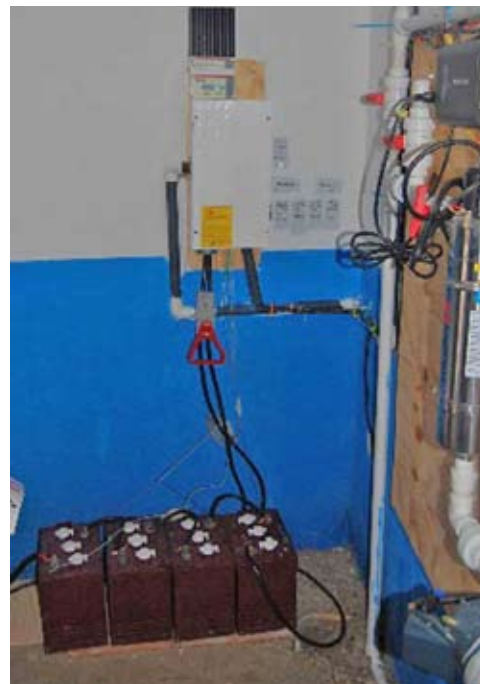
Inside, an array of batteries and electronic gear are distinguishing features
