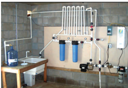
Standard LWW Filtration System
