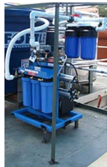
Compact RO unit purifies river water.
