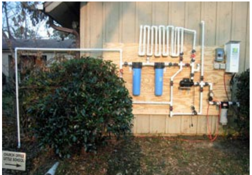
An outdoor water treatment system? Sure, if it's only going to be used for a short while and no other site seems suitable, as at Diamondhead Community Church near the Mississippi coast.
