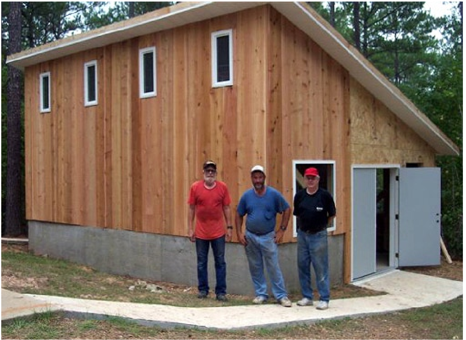
Proud of their handiwork at the newly-erected second water building on the Camp Hopewell Campus are (from left) Randall Swan, Roger Law and Buddy Nix, part of the team that spent a long weekend in construction.
